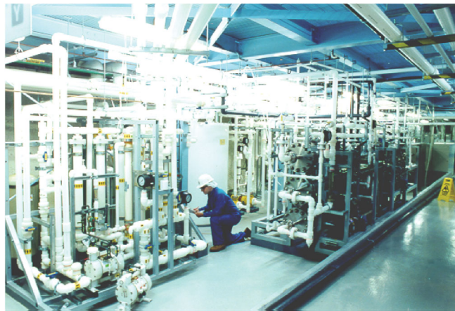
FIG. 7. Part of the water purification systems.
