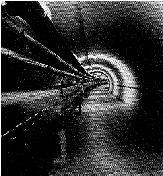
FIG. 2. The Main Ring accelerator tunnel magnets (Super-period A) bend the proton beam into a circle with a circumference of 6.2 km.
