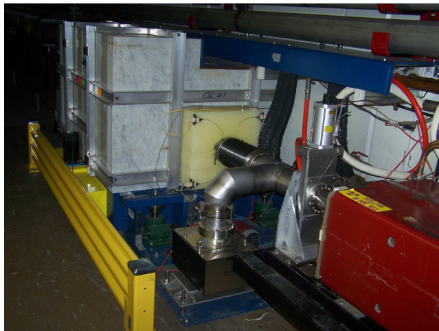
FIG. 7. One of four secondary collimators that employ a thick stainless steel vacuum chamber surrounded by a steel absorber to contain the shower particles. Radiation shielding for personnel is provided by 12 cm of marble placed on the top, ends, and aisle side of the collimator. At the upstream end a polyethylene block reduces neutron flux to upstream magnet coils. At the downstream end, masks are placed to absorb small angle outscattered particles.
