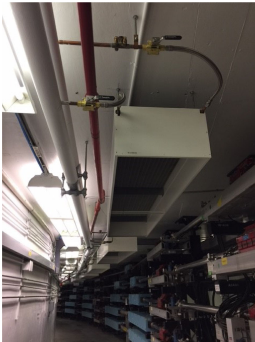
FIG. 48. Photograph of chilled beams of the air conditioning system next to the east arc magnets.
