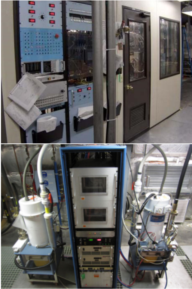
FIG. 36. The 20 kV high voltage enclosure and controls above and a pair of 10 kW IOTs with their controls below.
