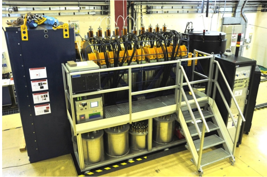
FIG. 1. Overall view of the 1 MV driver composed of ten stacked cavities in series.
